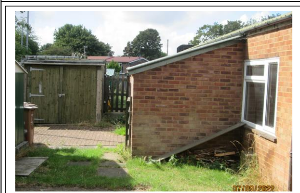
Photo 17 - Right side elevation with blocked down pipe gully
