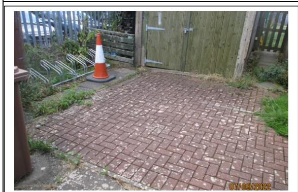
Photo 18 – Cracked and uneven paving slabs
