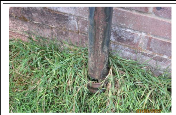
Photo 21 – Blocked don pipe gully
