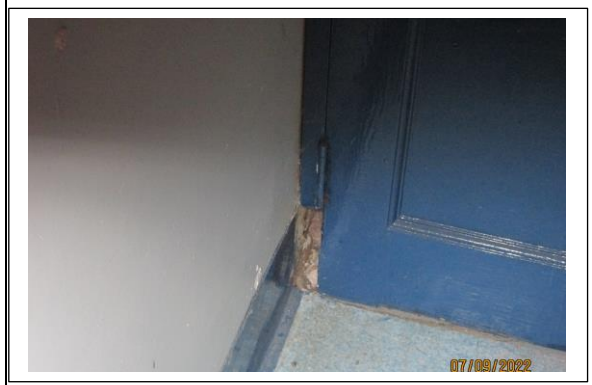
Photo 46 – Section of door liner missing
