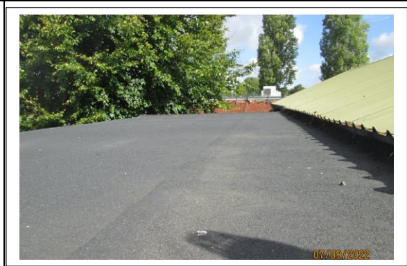
Photo 8 – Flat roof in reasonable condition . Cut edge corrosion to metal profile roof
