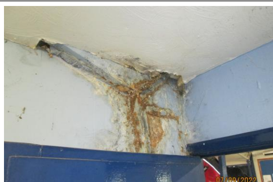
Photo 41 – Ceiling damage and corrosion to roof truss
