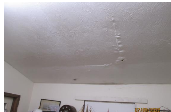
Photo 22 – Water damage to Artex ceiling
