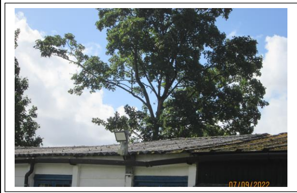
Photo 9 – Poor weathering detail at roof junction
