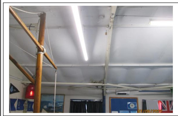
Photo 27 – Main roof truss out of alignment
