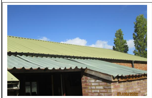
Photo 16 – Lean-to roof panels lifting and with cut edge corrosion.
