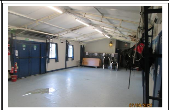
Photo 26 – Main hall. – Note puddles due to water leaks
