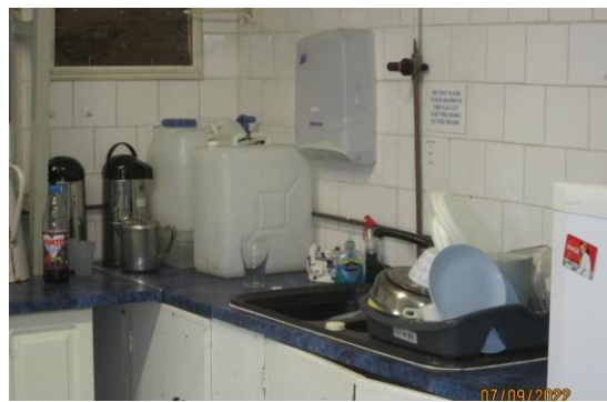
Photo 39 – Kitchen sink base unit cupboards damaged
