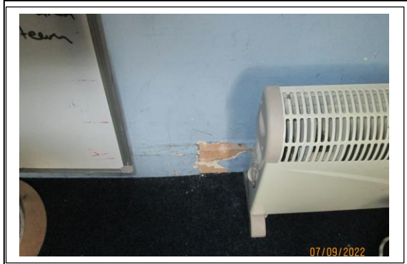
Photo 48 – Damage to skirting board
