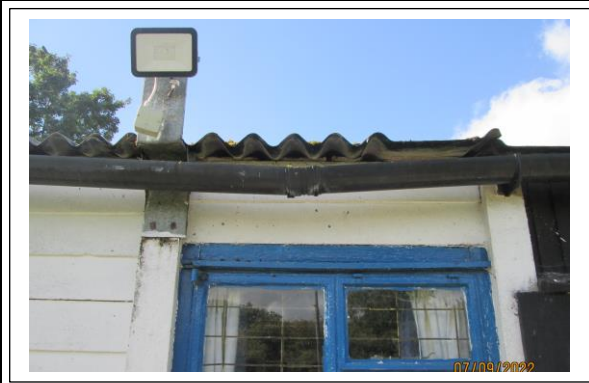
Photo 11 – Gutter unsupported and leaking
