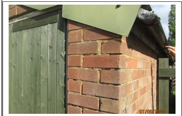
Photo 4 – Pointing to brickwork weathered with mortar joints falling out
