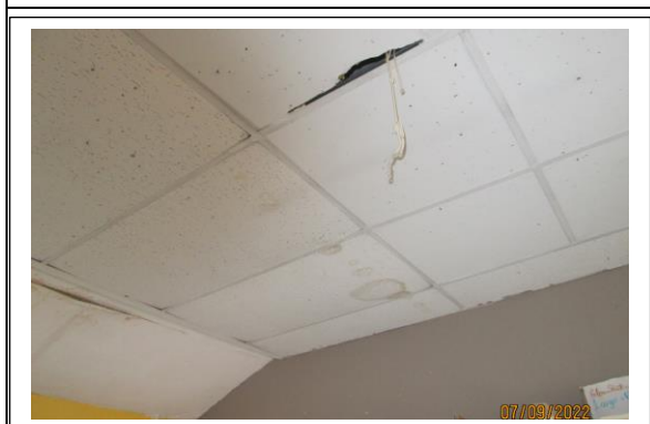
Photo 24 – Suspended ceiling in poor condition
