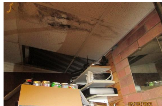
Photo 30 – Suspended ceiling tiles missing or water stained
