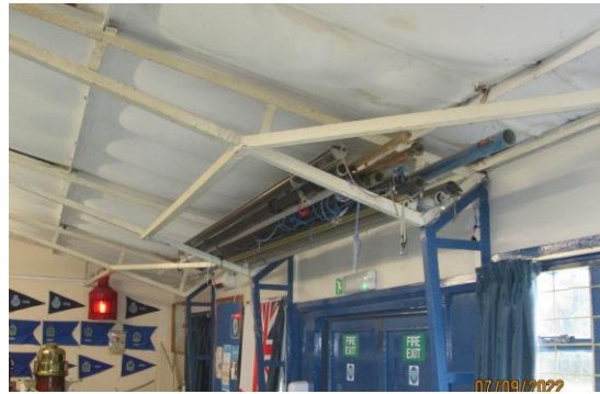
Photo 37 – Pipes stored between roof trusses creating additional imposed load
