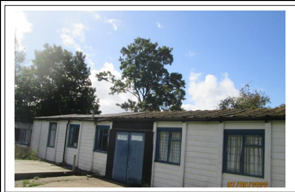
Photo 7 – Concrete wall panels with damp staining at low level
