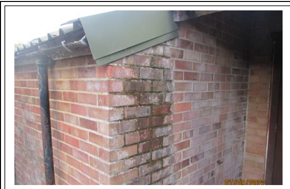
Photo 19 - Damp ingress to wall with deposition of salts over brickwork
