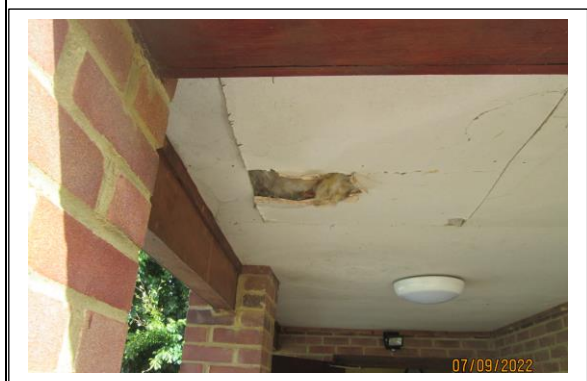
Photo 10 – Damage to ceiling in main entrance
