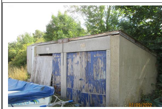
Photo 14 – Rotting timber doors and fascia
