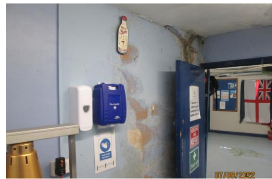
Photo 40 – Extensive damp ingress behind door causing plaster to de-bond
