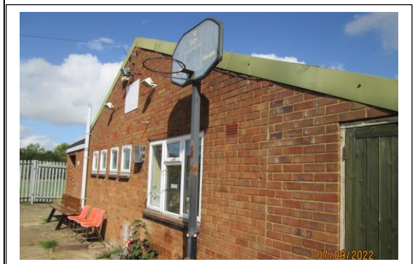
Photo 6 – High level brickwork pointing weathered.
