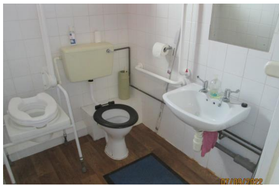
Photo 27 – Disabled toilet with non-contrasting grab rails
