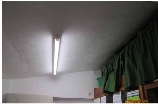
Photo 19 – Artex ceiling finish flaking
