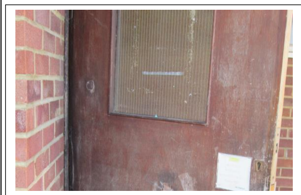
Photo 15 – Side door damaged and in poor decorative order
