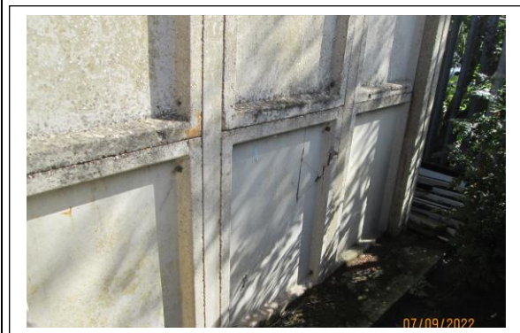
Photo 5 – Impact damage to pre-cast concrete panel
