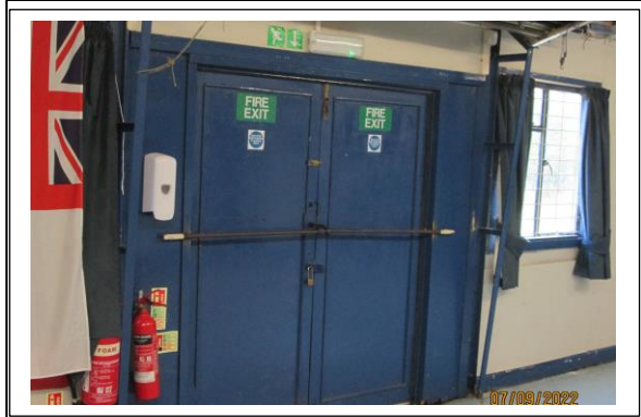
Photo 30 – Fire exit doors with obsolete panic bars
