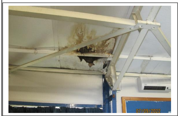
Photo 28 – Damaged ceiling panel and corrosion to steel truss
