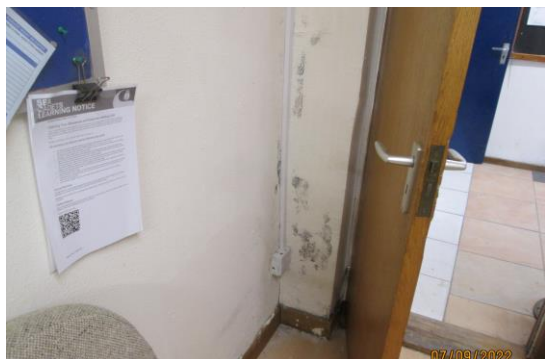
Photo 23 – Damp ingress to column and wall
