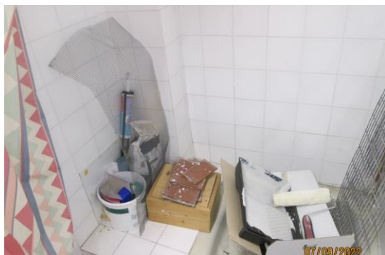
Photo 21 – Shower with tile damage
