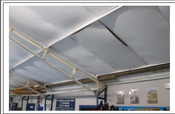
Photo 29 – Ceiling panels bowed and falling out
