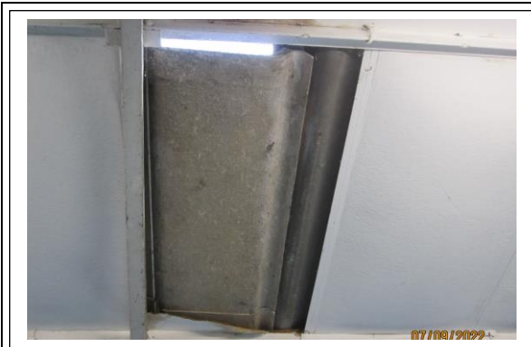
Photo 31 – Large gap in main roof
