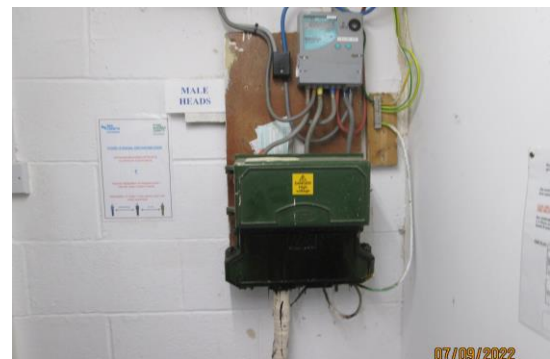
Photo 24 – Electric supply head leaking bitumin due to overheating
