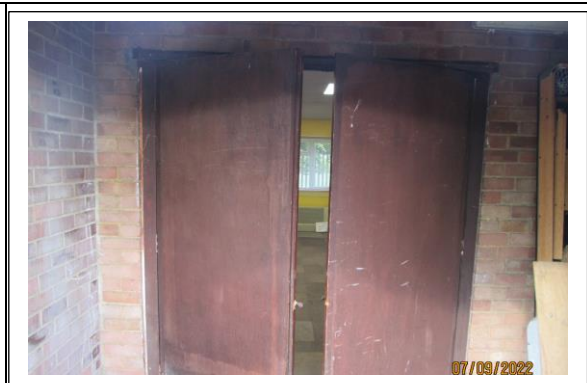
Photo 20 – Fire exit doors damaged and in poor decorative condition.
