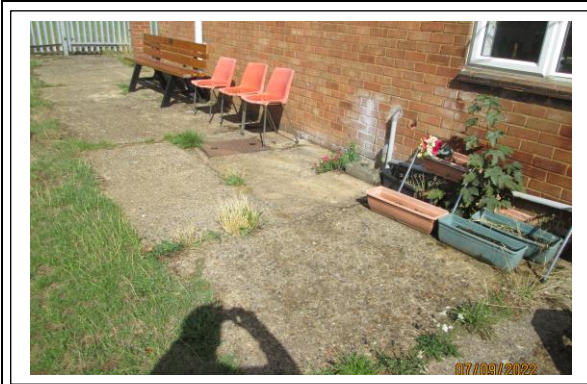
Photo 7 – Staining to wall and brickwork damage at low level
