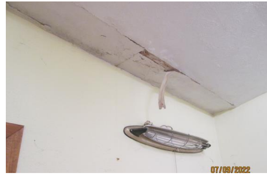
Photo 20 – Ceiling edge detail falling away due to water ingress
