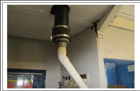
Photo 47 – Rainwater pipe diverted across access route
