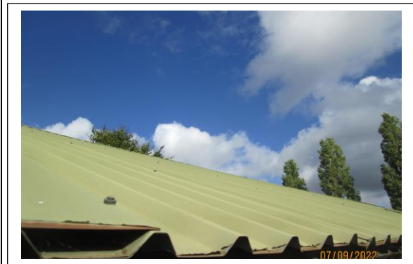
Photo 3 – Profile metal roof with cut edge corrosion
