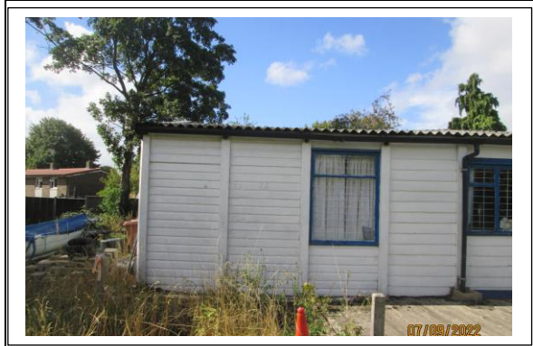
Photo 12 – Concrete panels damaged
