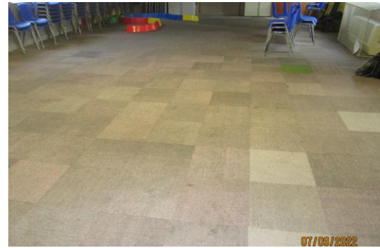
Photo 26 – Carpet tile floor covering marked and dirty with inconsistent tile colour.
