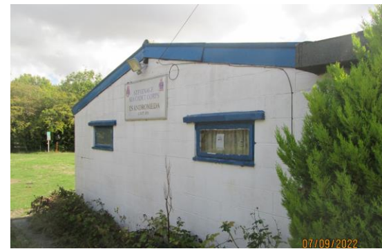
Photo 4 – Blockwork cracked adjacent to window
