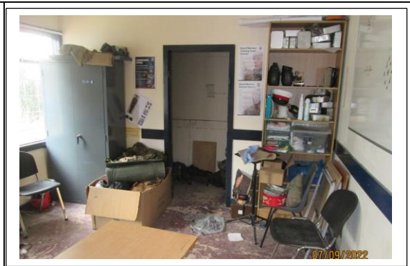
Photo 44 – Storage room door removed and floor uneven with paint worn
