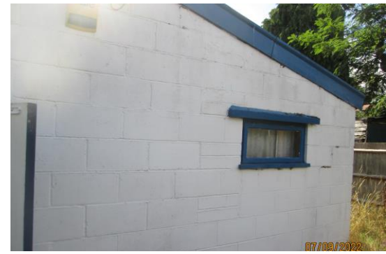
Photo 2 – Mortar joints to blockwork cracked and falling out.
