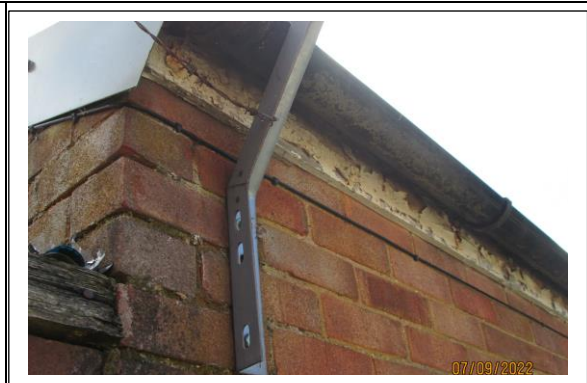
Photo 14 – Fascia in poor condition and rotting to wall plate
