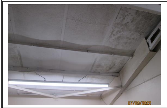
Photo 34 – Ceiling panels water stained and bowed
