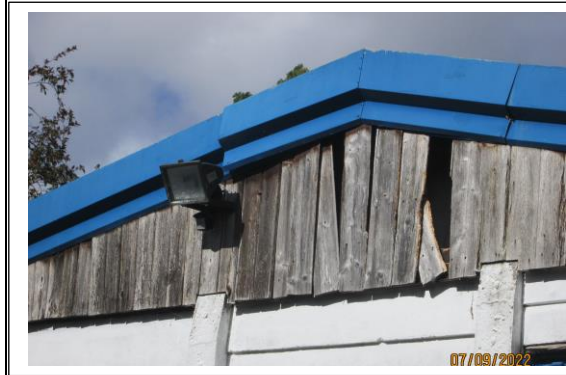
Photo 16 – Timber cladding rotted and falling out
