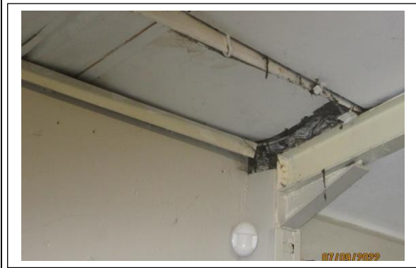
Photo 33 – Evidence of water ingress at eaves
