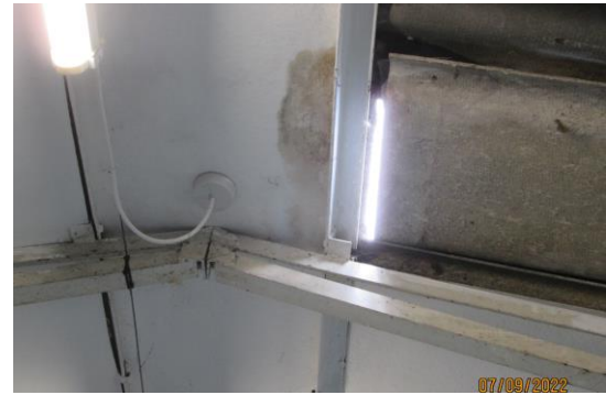
Photo 38 – Electric light ceiling rose close to area of water ingress
