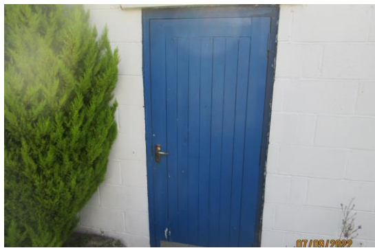
Photo 3 – main entrance door with rotting at low level
