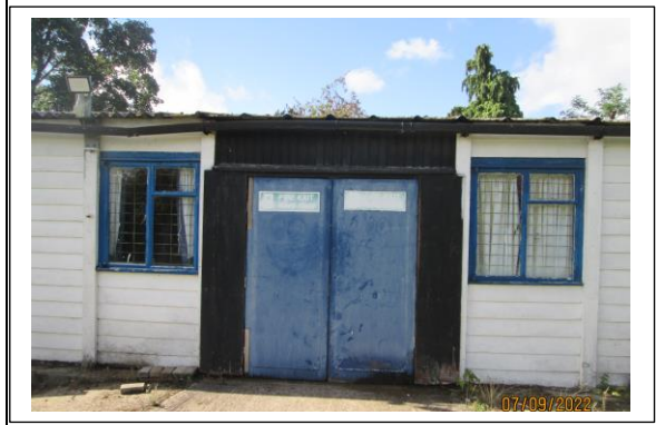
Photo 10 – Fire exit doors and timber panels rotting at low level
