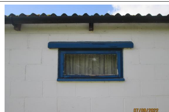
Photo 6 – Cracked glazing to window
