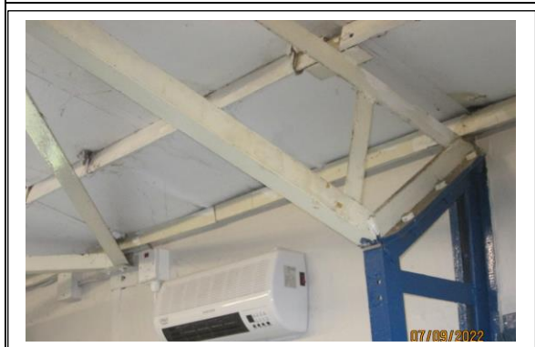
Photo 36 – Electrical heater and spur position below leaking roof
