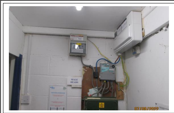
Photo 25 – Main electric meter and boards with loose cables
