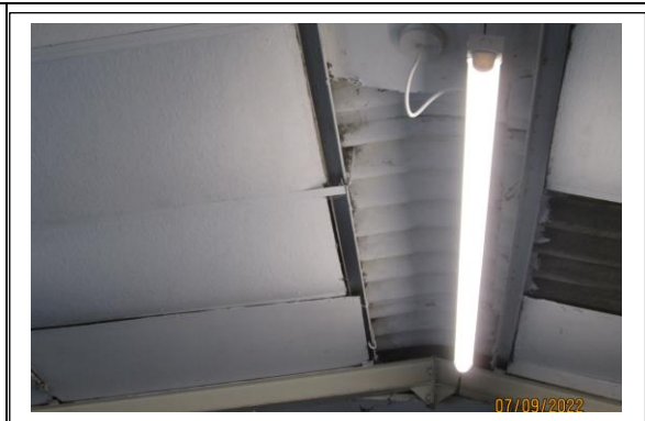
Photo 32 – Evidence of water ingress below ridge detail
