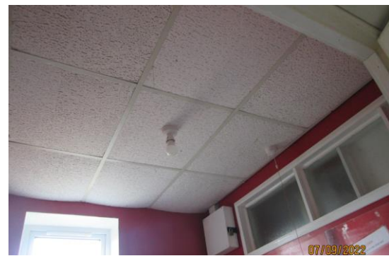
Photo 28 – Suspended ceiling with tiles bowed
